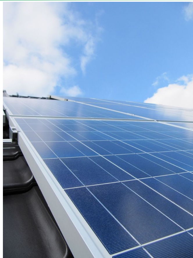
Solar panel installed on the roof of a building
